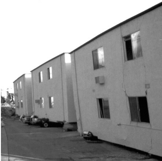
Fig. 1: Collapsed Tuck-under Parking
