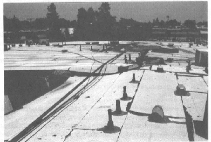
FIG. 7. Failed Roof Diaphragm at L-Shaped Intersection
